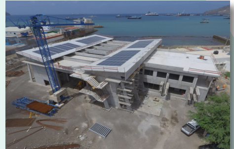
Ocean Science Centre Mindelo under construction on the Cape Verde archipelago in the tropical North Atlantic. Photo credit: Filipe Mandel.
